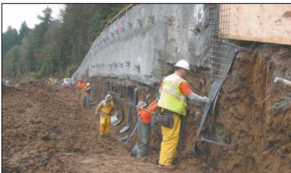
The contractor continues to install soldier piles, soil nails, drainage and shotcrete on the retaining walls north and south of the Sellwood Bridge. Macadam Avenue (Highway 43) traffic lanes will shift west along the new walls in January. (Photo courtesy of Mike Pullen, Multnomah County)
