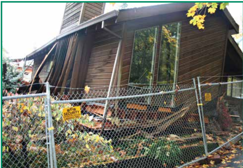
This photo taken on November 9 shows one of the homes damaged in the Terwilliger landslide. (Post photo by Polina Olsen)
