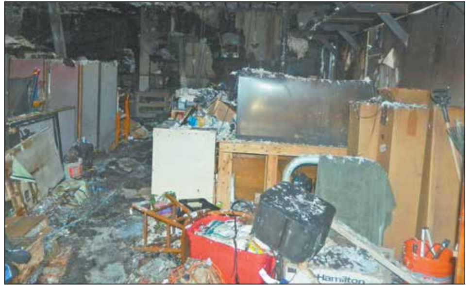
Fire damaged the Coin Cottage on Sept. 9. (Post photo by Erik Vidstrand)
