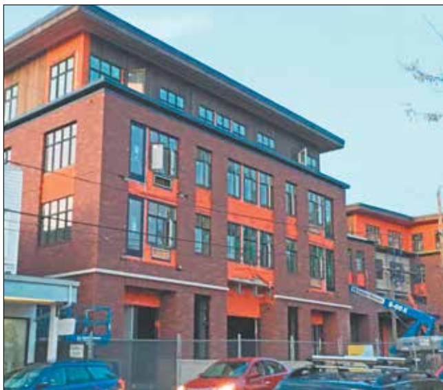
Bremik Construction expects to complete the Multnomah Village Apartments by late fall. (Post photo by Erik Vidstrand)
