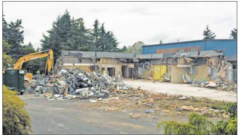
Bremik Construction demolishes the former Children's Center at Southwest 33rd and Capitol Highway. Multnomah neighbors have dubbed the planned 71-unit, four-story building to be constructed on this site as "the tower," a symbol of the association's opposition to high-density infill. (Post photo by Erik Vidstrand)
