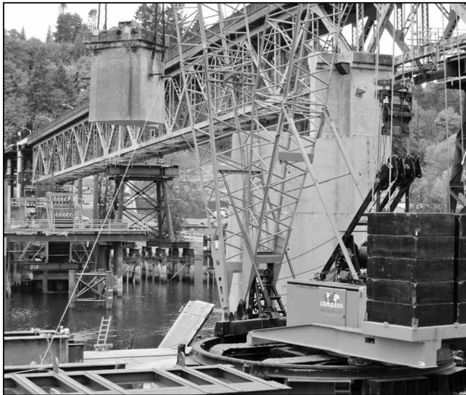
A crane removes a 300,000 lb. chunk of concrete from Pier 2. (Photo courtesy of Mike Pullen, Multnomah County)
