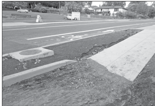
Mud covers the new sidewalk at the corner of Southwest 37th Avenue and Vermont Street after a two-hour cloudburst on Sept. 1. The ground is higher than the sidewalk in that area. (Photo courtesy of Rose Florek)
