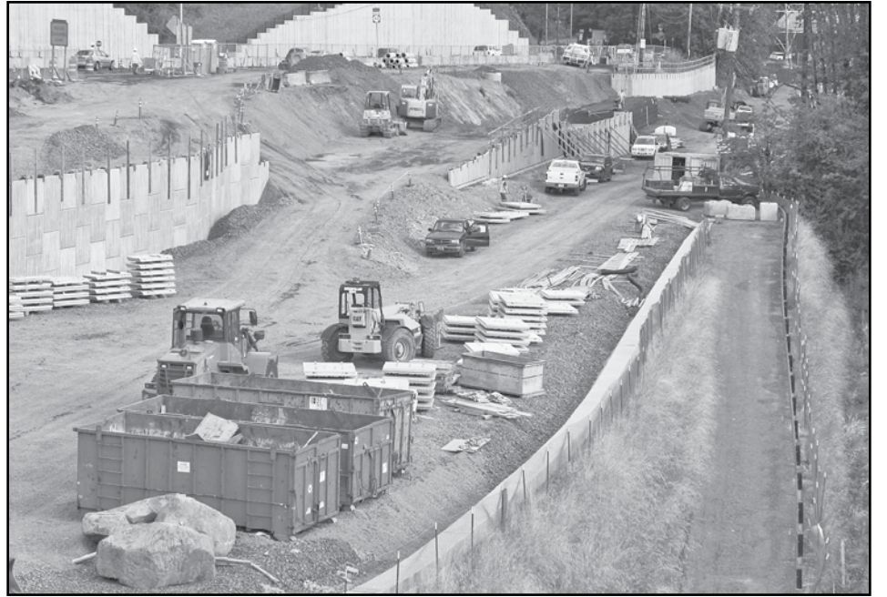
Many types of retaining walls are taking shape north of the Sellwood Bridge. (Photo courtesy of Multnomah County)
