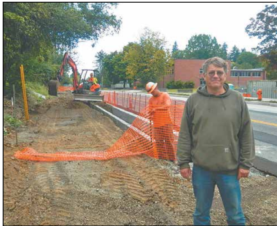
Jim Peterson has been building relationships with the contractors at the Multnomah Boulevard construction project. He lives and works in the heart of the construction zone. "The crews have been fantastic," Peterson said. "It's the city you need to watch out for!" (Post photo by Erik Vidstrand)
