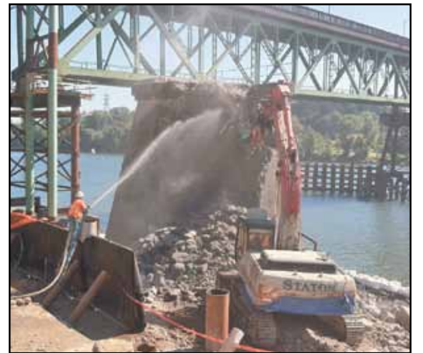
A Sellwood Bridge worker sprays a stream of water at one of the old west piers in July as a way to help control concrete dust during demolition. (Photo courtesy of Mike Pullen, Multnomah County)
