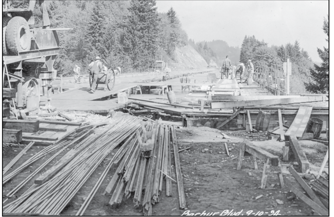
Builders construct the original Vermont Street Bridge along Southwest Barbur Boulevard in September 1934. (Photo courtesy of Oregon Department of Transportation)
