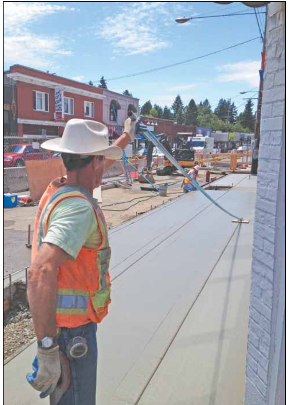
City contractors taking advantage of a dry day in June to pave one of the new sidewalks in the village. (Post photo by Erik Vidstrand)
