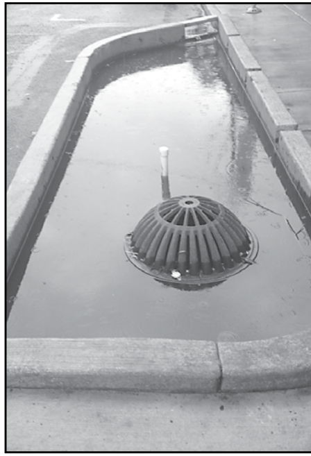
This bioswale located on Southwest Capitol Highway at 36th Avenue isn't draining properly.
