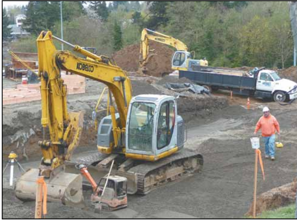
A new Walgreens drugstore is under construction along SW Capitol Highway near Barbur Blvd. (Post photo by Jillian Daley)
