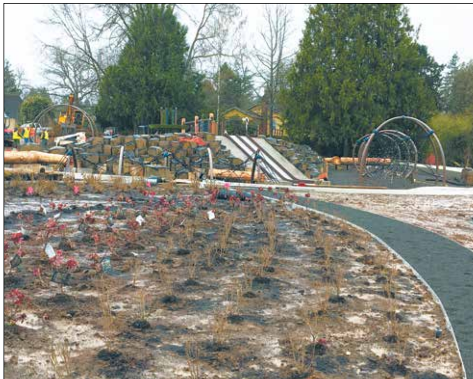
Spring Garden Park is currently under construction but should be opening in late May or early June. (Photo courtesy of Portland Parks and Recreation)
