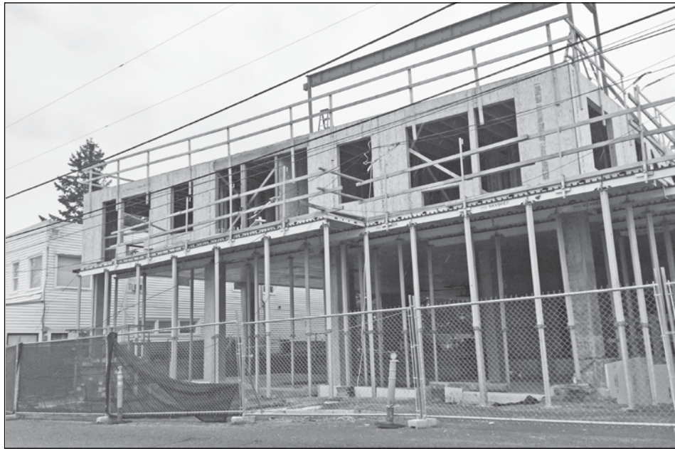
One infill project that has the land use committee concerned is the 70-unit, four-story apartment building under construction on Southwest Capitol Highway at 33rd Avenue in Multnomah Village. (Post photo by Erik Vidstrand)
