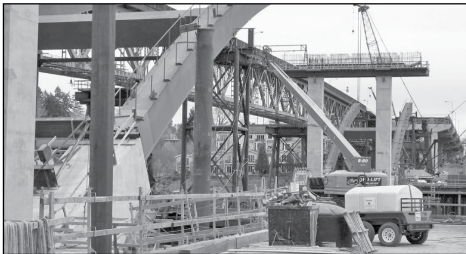
The east and center arch span segments on the new Sellwood Bridge are installed in sequence designed to load the weight evenly between the two spans. (Photo courtesy of Multnomah County)
