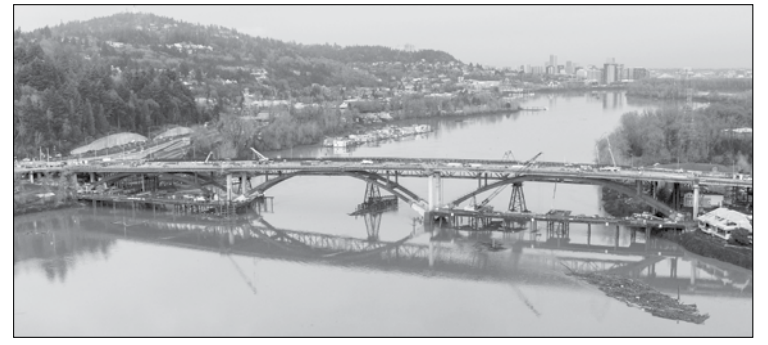
Aerial view of the new Sellwood Bridge as it appeared in January. (Photo courtesy of Multnomah County)
