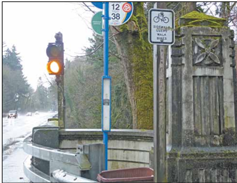
The Vermont bridge is located along Barbur Boulevard at Southwest Parkhill Drive. (Post photo by Jillian Daley)
