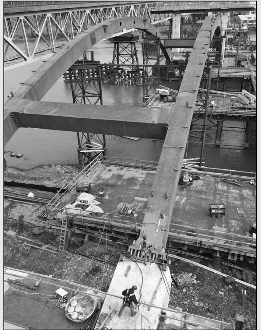
The contractor for the Sellwood Bridge continues to install cross braces between the two steel arches of Span 3, at the west end of the Sellwood Bridge. Workers are installing 3,000 bolts at each connection in the arch segments. (Photo courtesy of Multnomah County)
