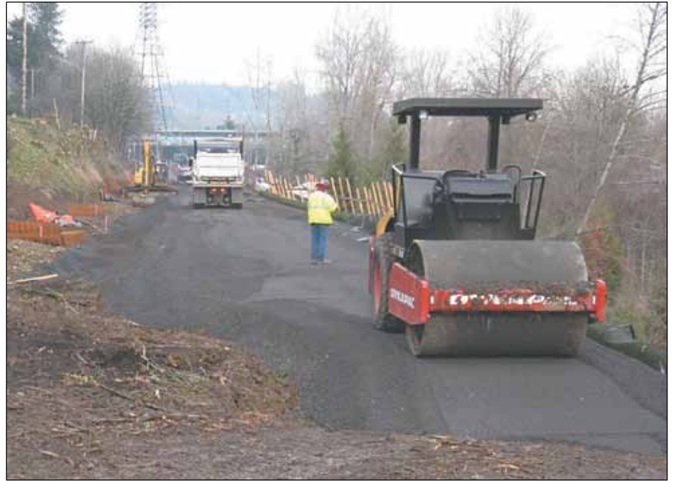
Sellwood Bridge workers pave the new trolley corridor on the west side of the Willamette River in early January. (Photo courtesy of Multnomah County)
