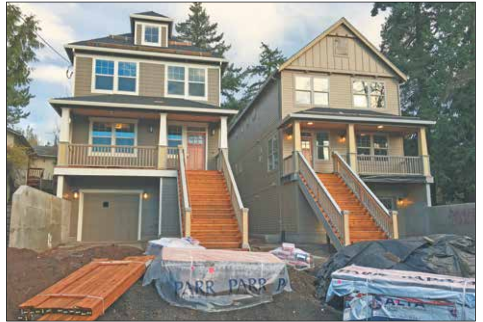
Where one old house used to rest on a large lot, it was demolished and now two houses near completion. (Post photo by Erik Vidstrand)
