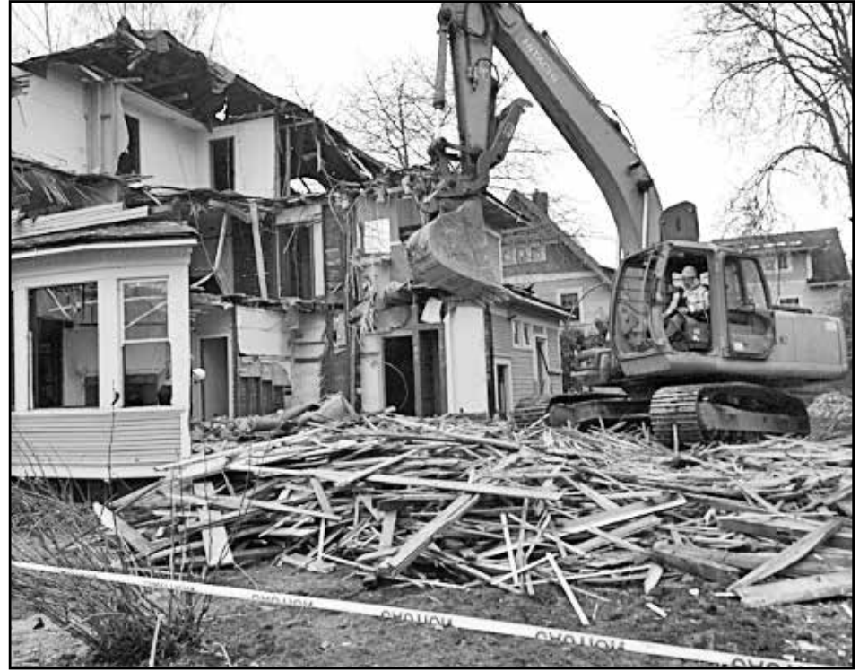
The Hillsdale Neighborhood Association wants the city of Portland to form a task force to review homes slated for demolition by developers. (Photo courtesy of bikeportland.org)
