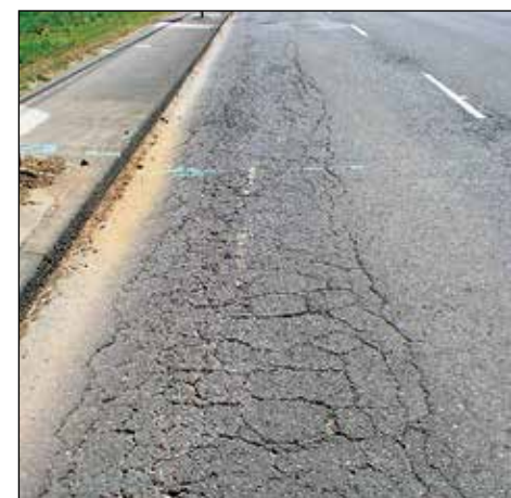
Arterial in poor condition
